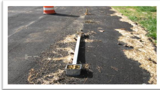
Fractured Anchor between Post 1 and 2
